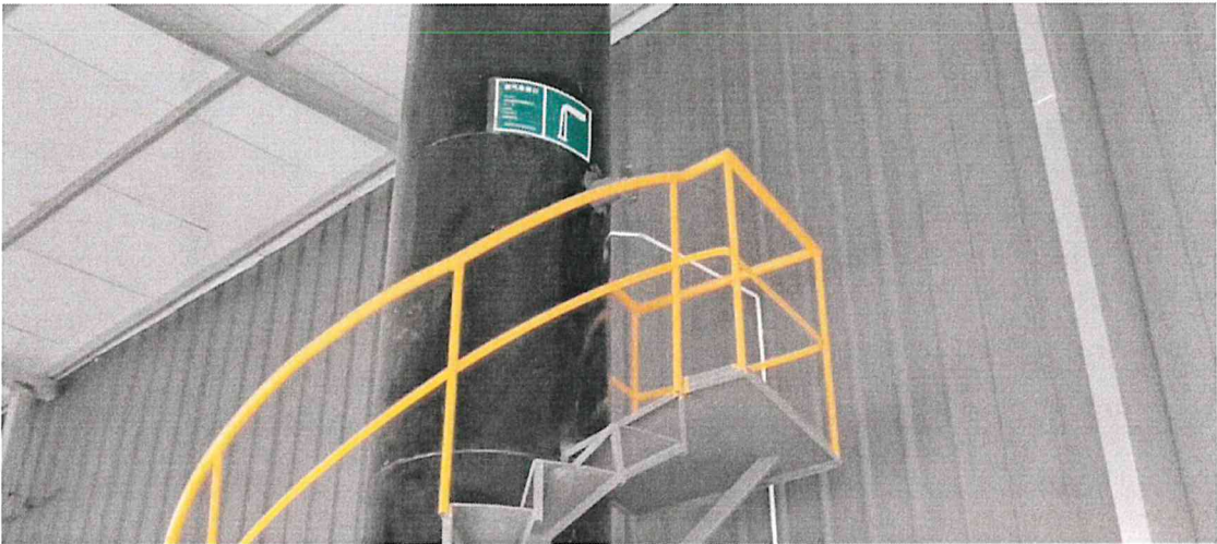
P5 喷涂底漆工序排气筒
